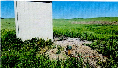
Well and pump house
