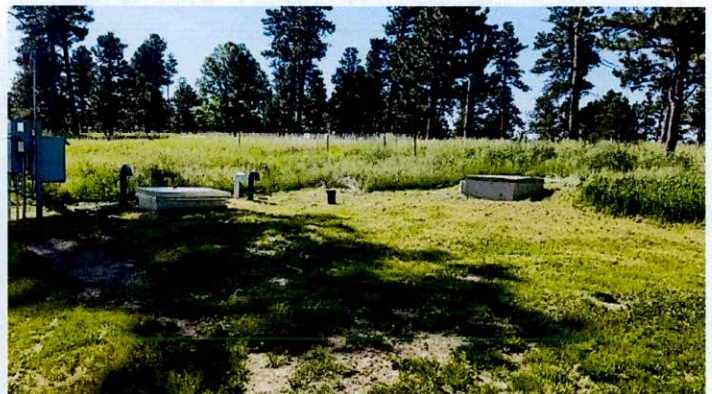
5,000 gallon storage to right, booster pit to left
