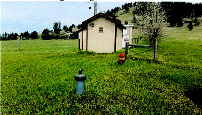
Well and pump house
