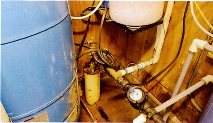
2005 well inside utility room/shower house
