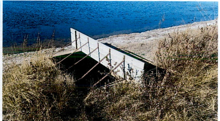
riser and trash rack
