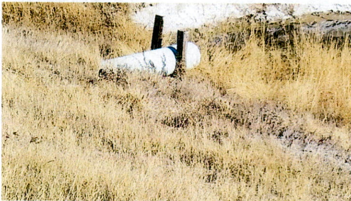
PVC principal spillway outlet
