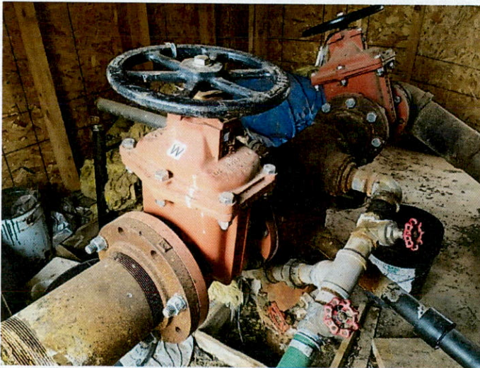
Well and associated plumbing
