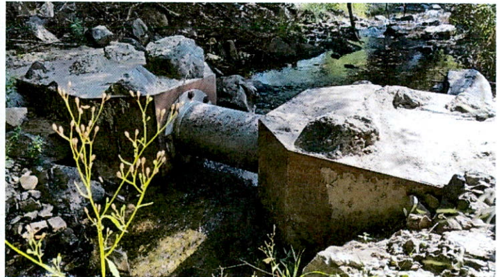
Blacktail Water Treatment Plant discharge to Deadwood Creek
