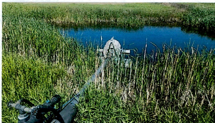
Diversion point (pump intake and trash screen in dugout)
