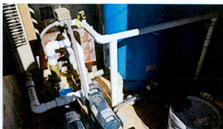
Pumps and appurtenances
