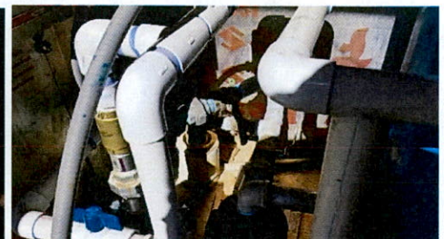
Well head in photo center
