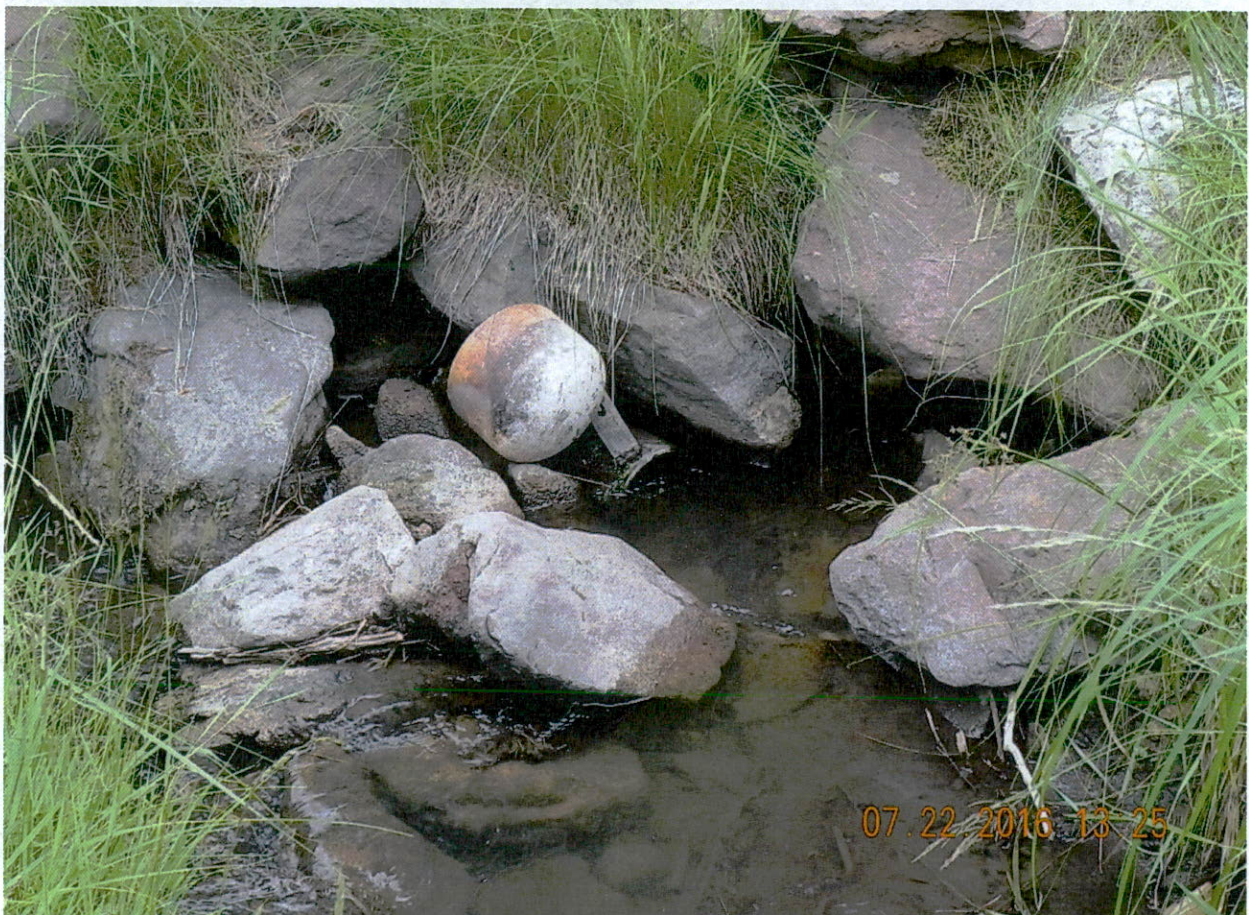
Photo 2 Inlet pipe on Elk Creek.
