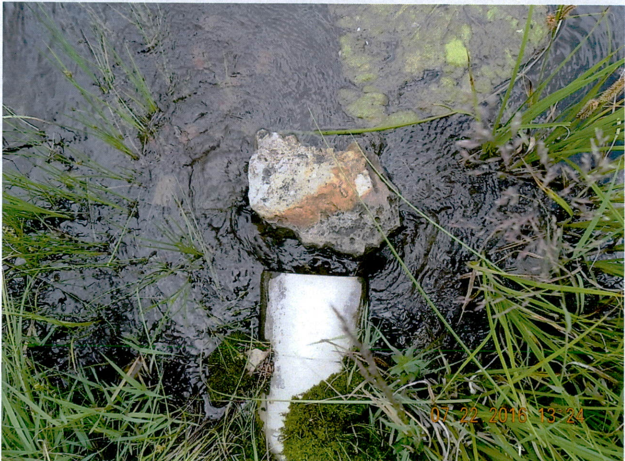
Photo 4 Inlet pipe flow into the pond.
