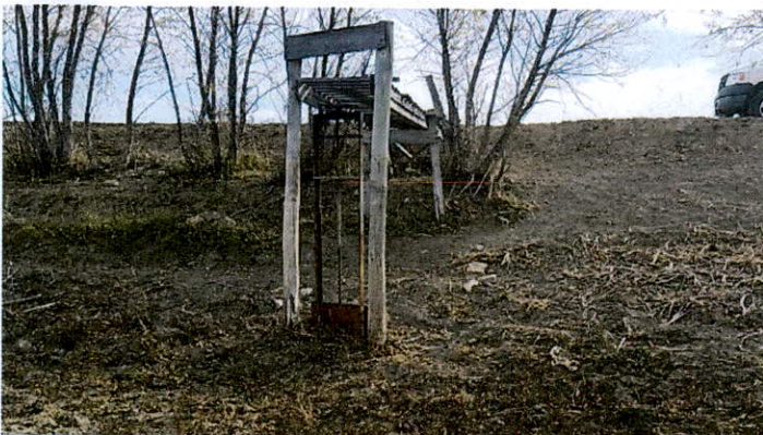
by-pass spillway with slide gate with hand wheel
