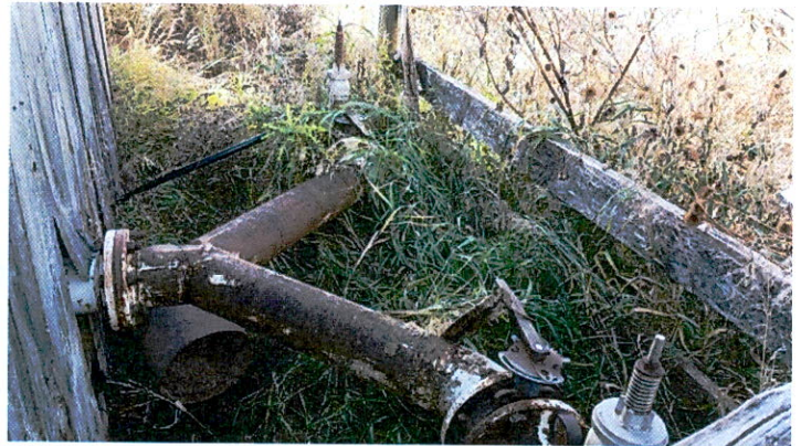
piping and valves to north and south pipelines
