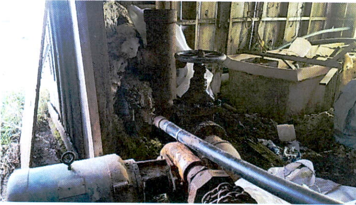
well, pump and associated plumbing
