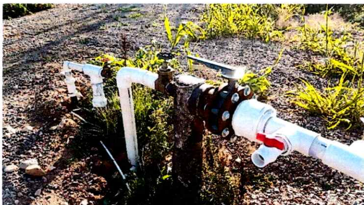
west well with replaced valves and plumbing
