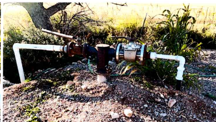
east well with replaced valves and plumbing
