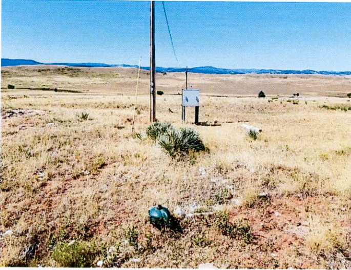
well and control panel
