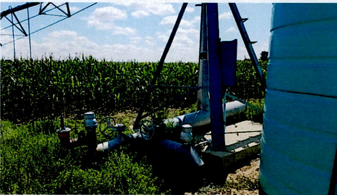
Appurtenances at pivot, gravity flow from BFID
