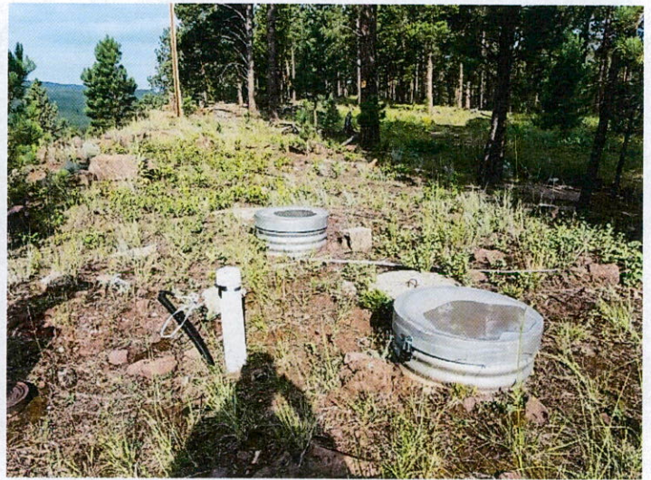
Twin 1,200 gallon concrete storage tanks
