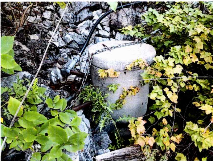
spring Box and piping
