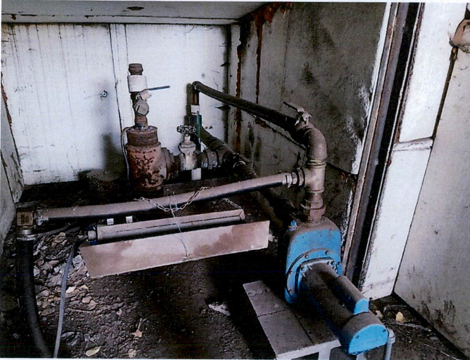
well and booster pump
