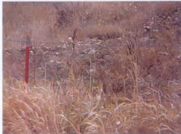
Photo #6 Ditch plugged with gravel.
