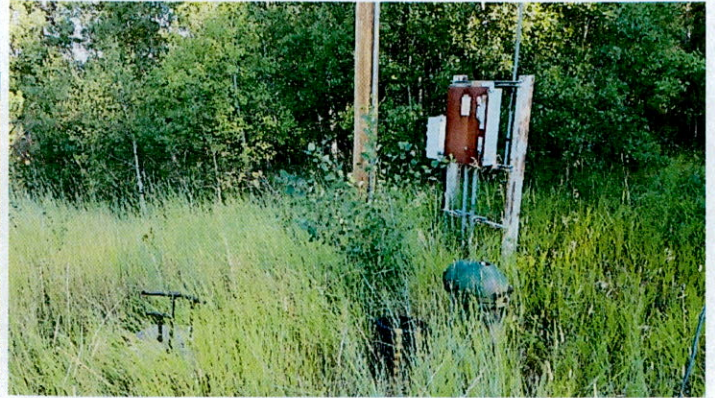
Water Supply Well WS-8
