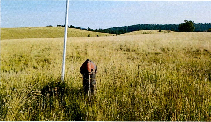
Water Supply Well WS-2
