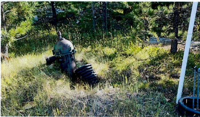
Water Supply Well SW-15
