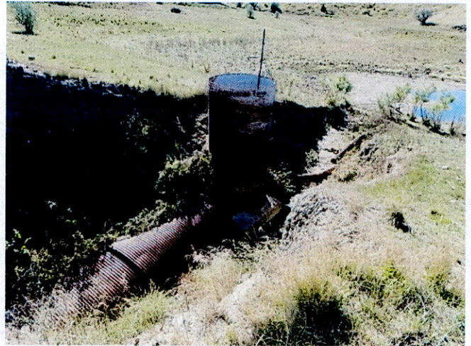
riser and barrel of large dam (breached)
