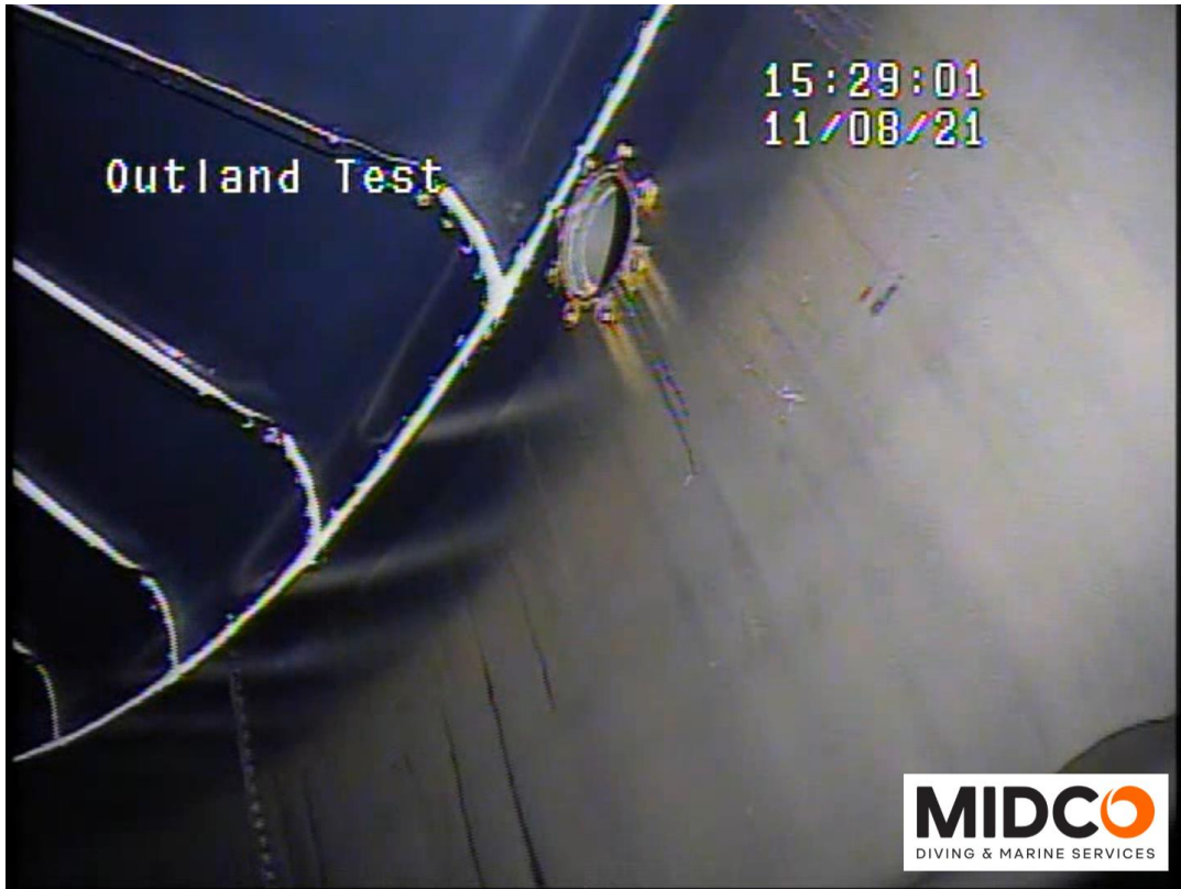
Wall to Roof Seam and Overflow – Corrosion Noted
