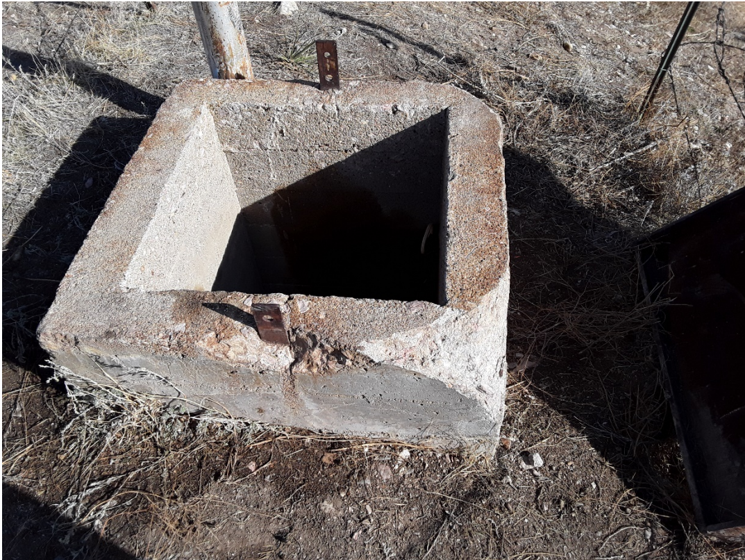
Access Hatch – Spalling Noted
