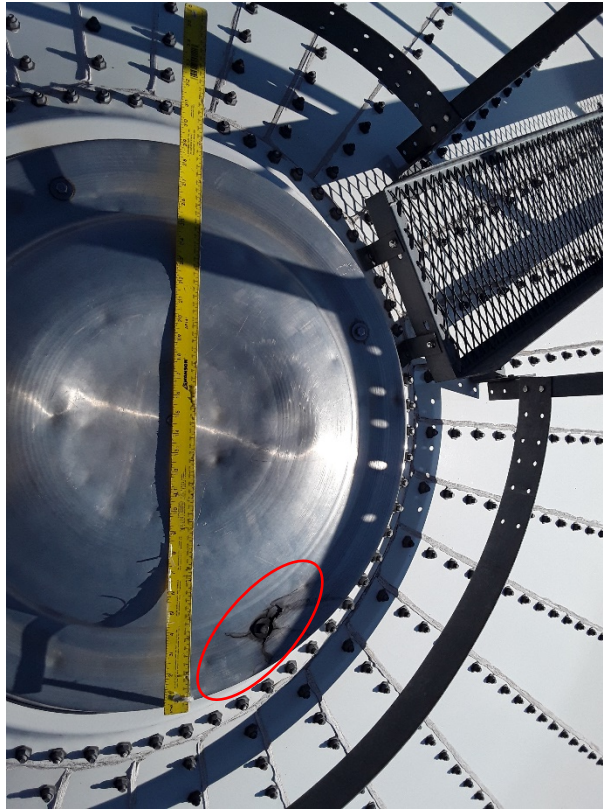
Roof Vent – Deterioration Noted
