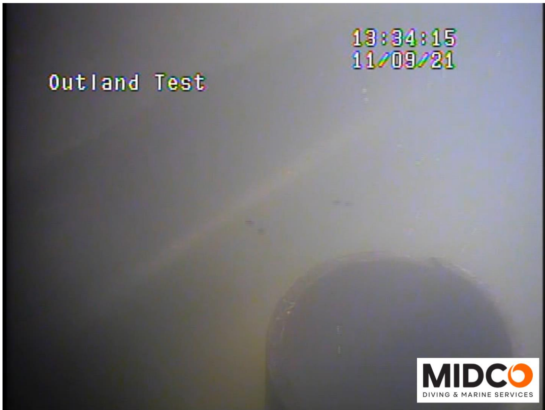
Common Inlet/Outlet – Corrosion Noted
