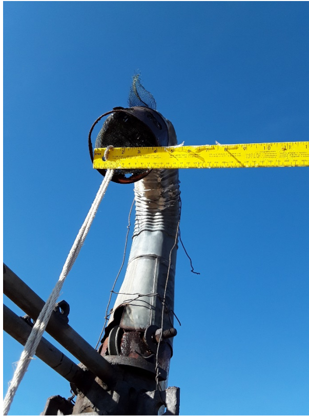
Roof Vent – Deterioration Noted
