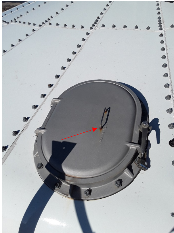
Access Hatch – Hardware Corrosion Noted
