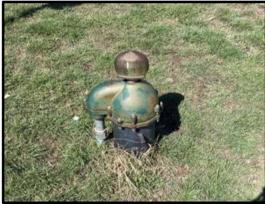
Figure 3.4.1-1: Well #2 (Not in Use)
