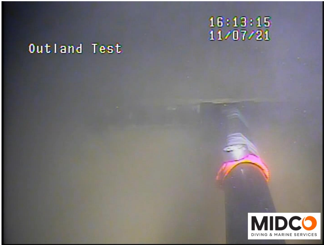
Cleaning Reservoir – High Turbidity Noted Upon Entry
