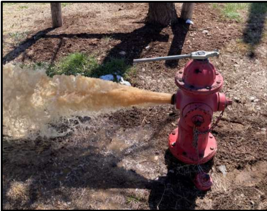
Figure 3.1-2: Hydrant near Intersection of Elm and 4 th St
