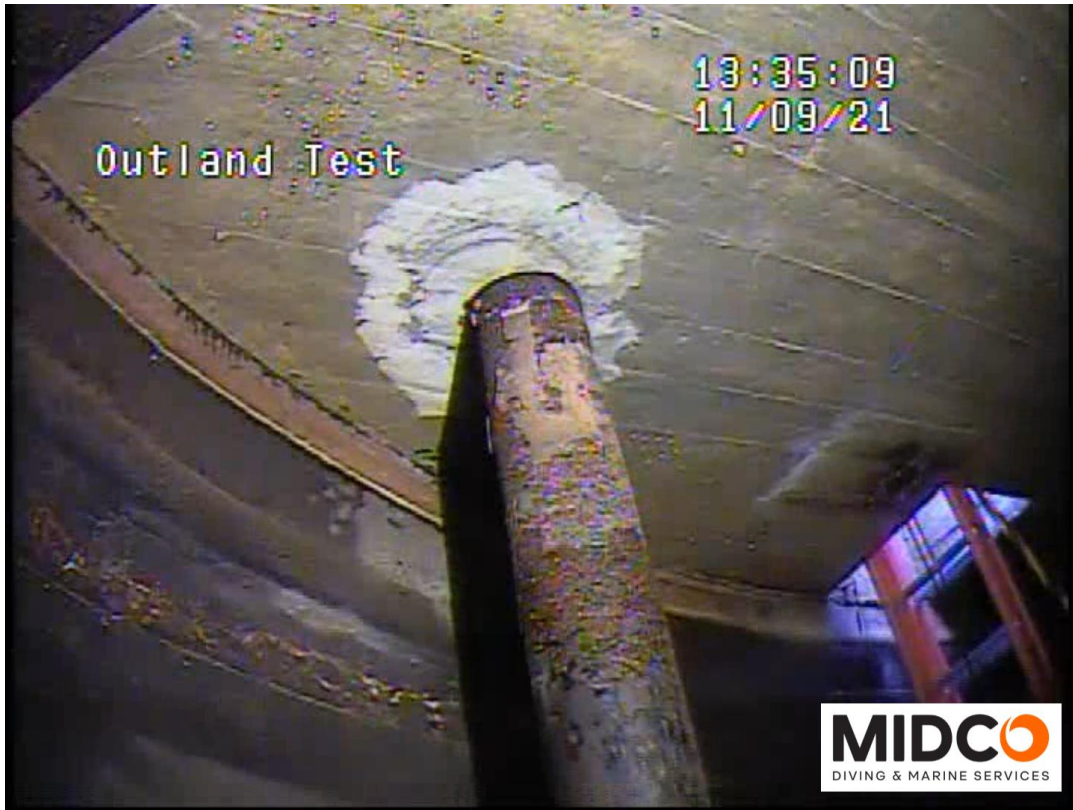
Overflow Plumbing – Corrosion Noted
