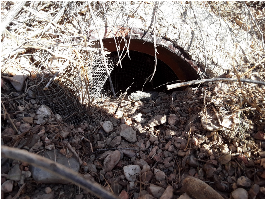
Overflow Plumbing and Screen – Screen Deterioration & Debris Noted
