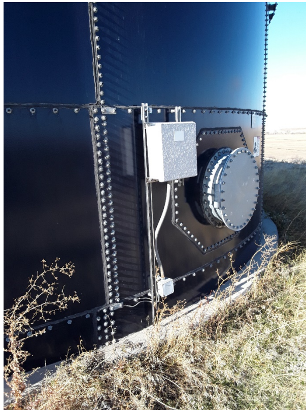
Exterior Telemetry and Man Entry
