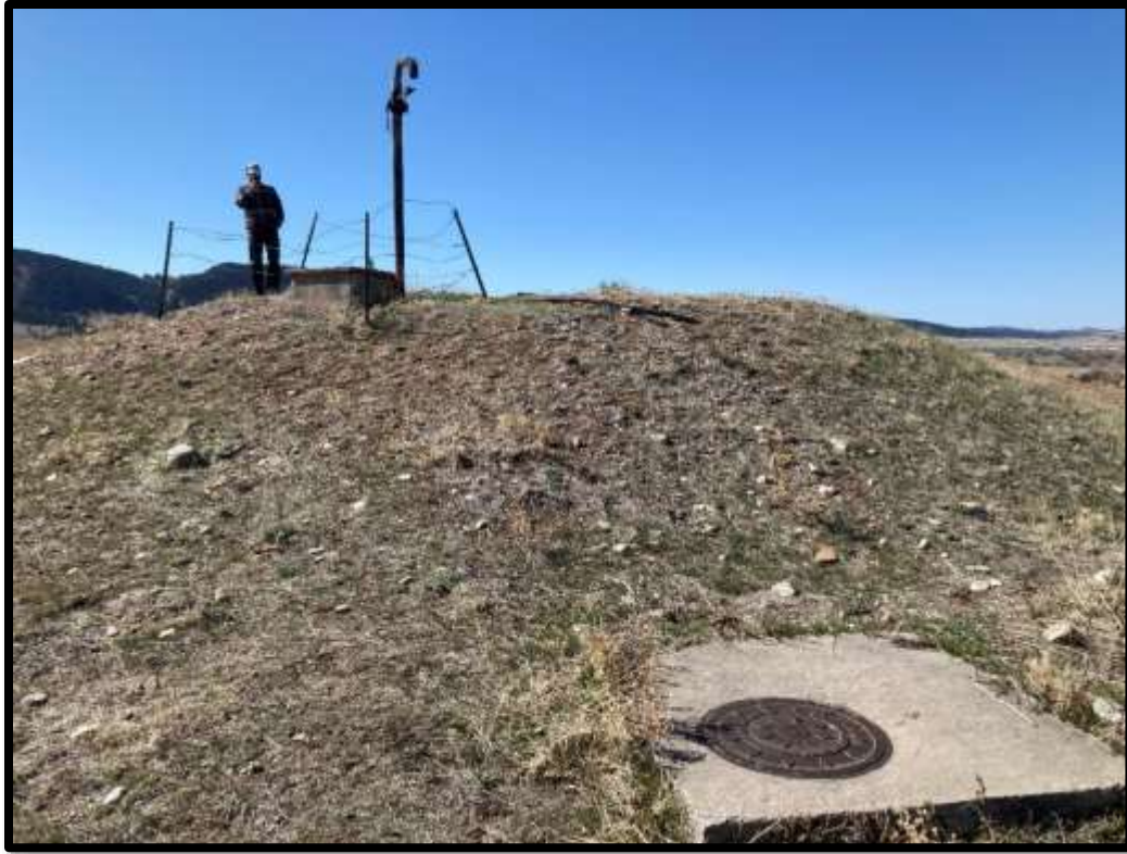
Figure 3.5-2: Underground Storage Tank
