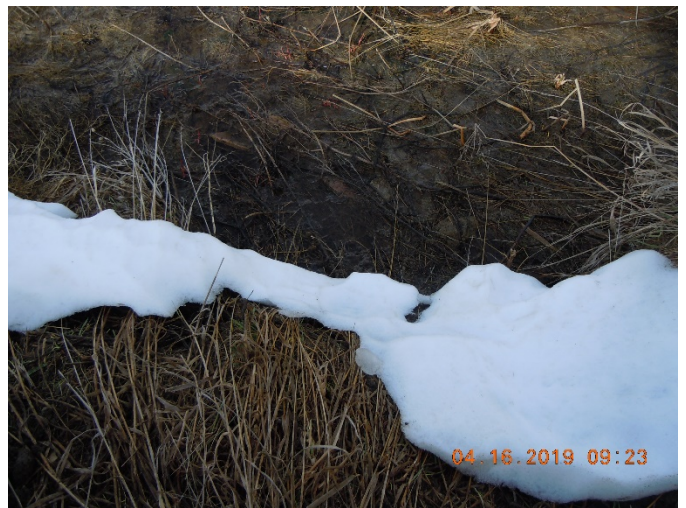
Figure 16: Erosion on Cell #4
