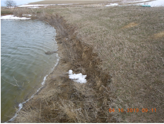
Figure 10: Erosion on Cell #4
