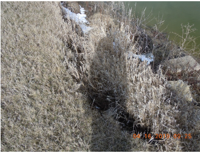
Figure 17: Erosion on Cell #4
