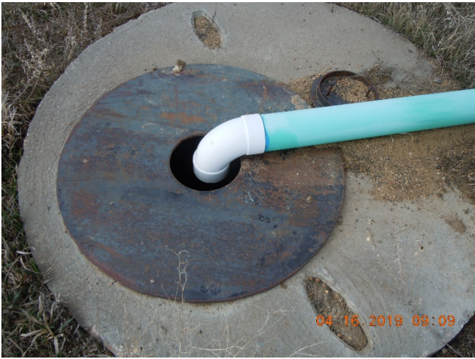
Figure 6: Transfer Pipe to Cell #4
