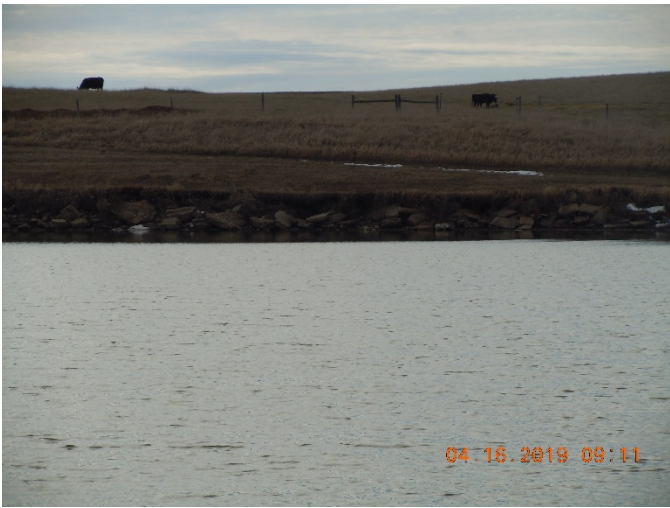
Figure 11: Erosion on Cell #5 Facing East
