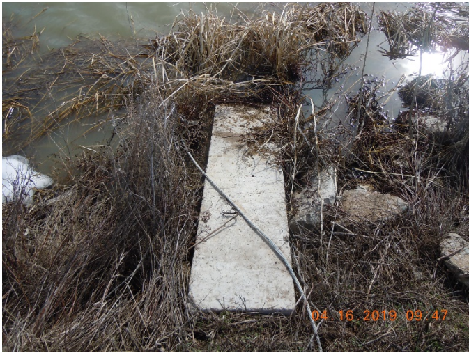
Figure 21: Depth Indicator in Cell #3 without markings
