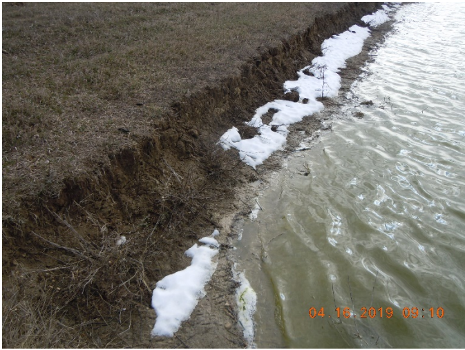
Figure 9: Erosion on Cell #4
