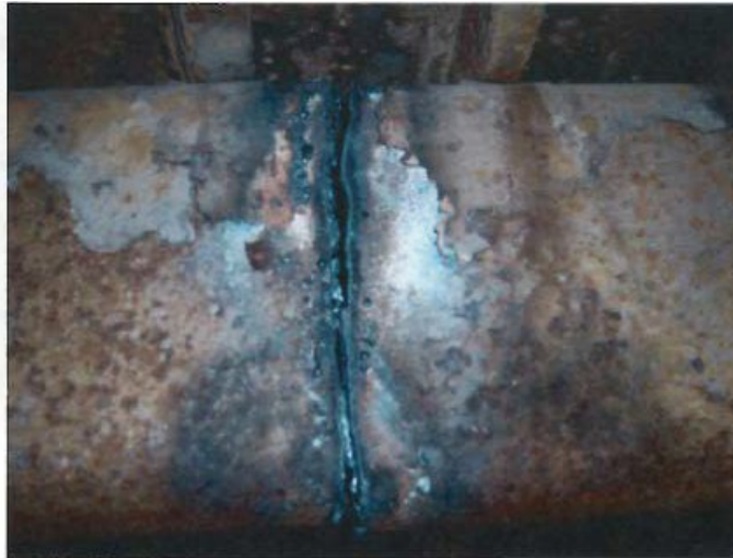
Photo #4: Chassis rail cut in half
