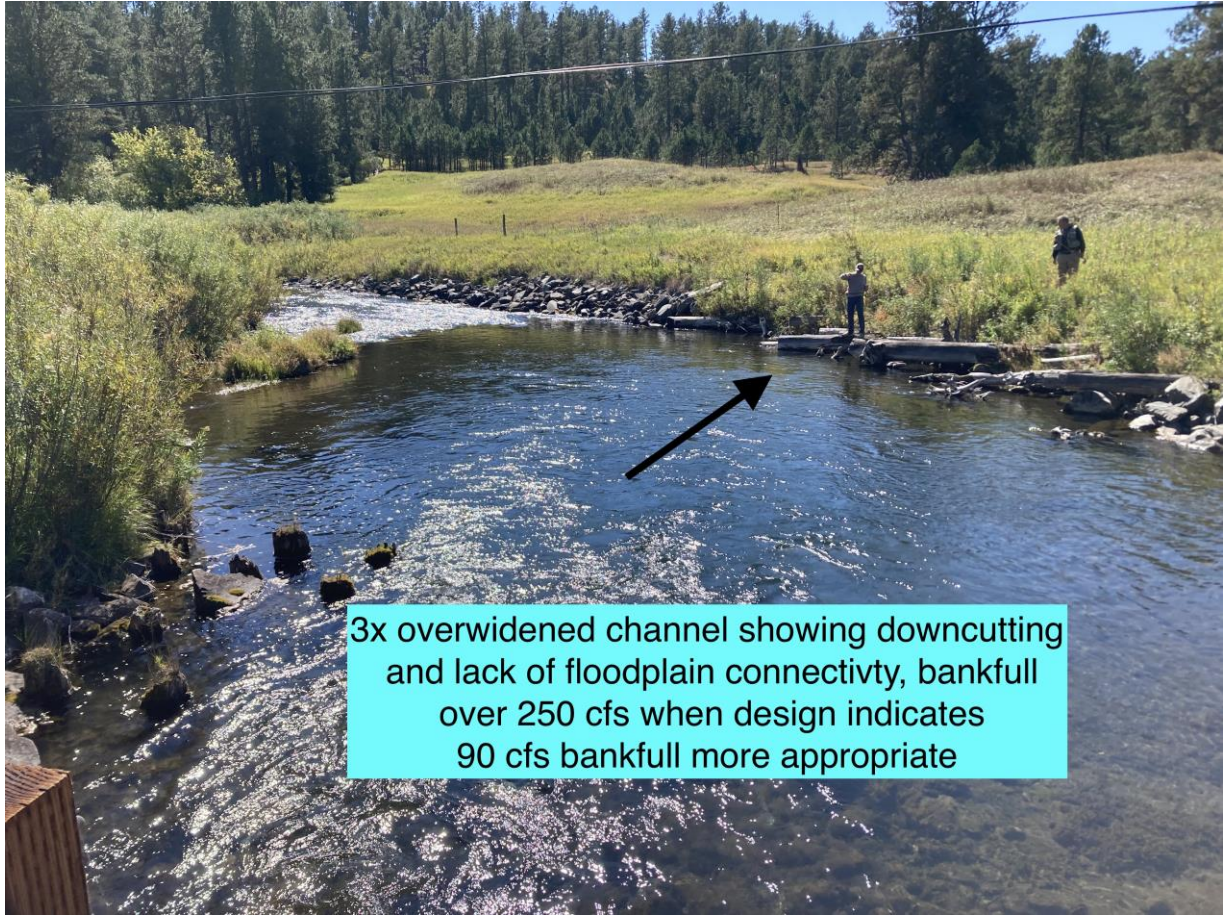
Figure B4. Photo from September 2024 showing 3x overwide channel, evidence of downcutting/erosion of channel banks and lack of floodplain connectivity.
