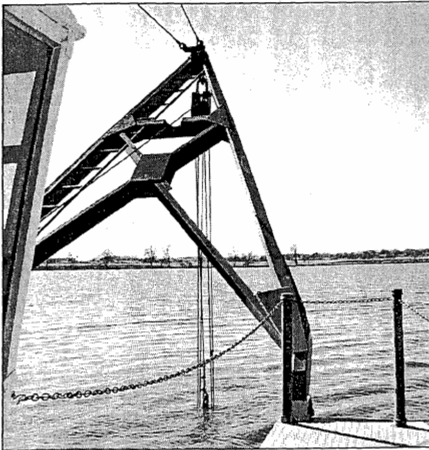
This shows the beam which holds the cutter and cables while the cutter is below the water digging through the silt.
