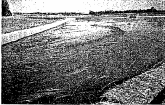
The cell of the holding ponds with water and silt in it. You can see how the bales are covered with burlap.
