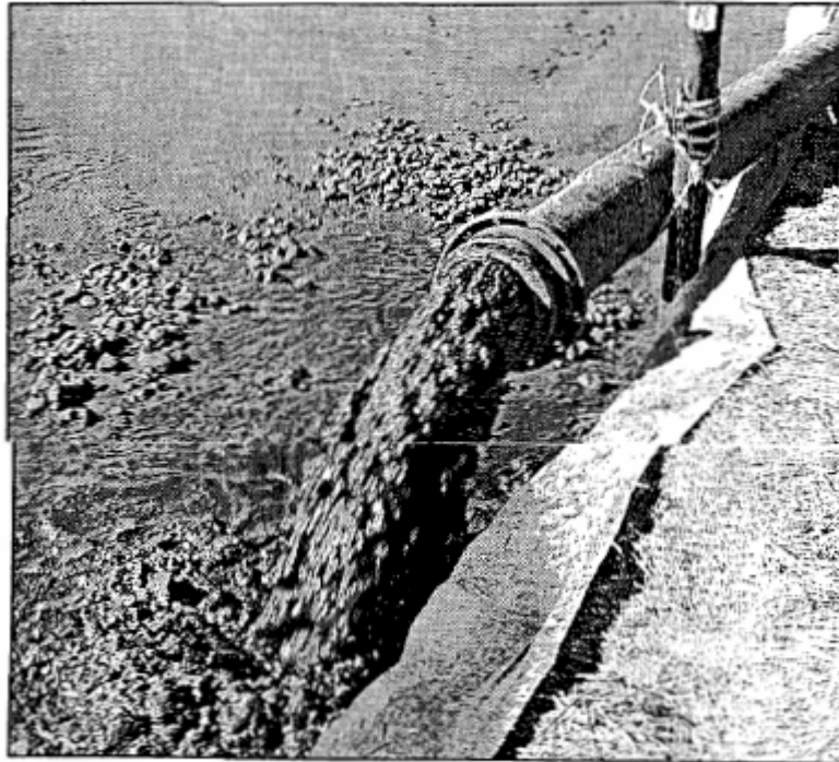
The discharge of 30% sediment and 70% water, as it runs out of the pipe attached to the dredge and into the holding ponds.
