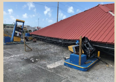
Destroyed dispensers after Hurricane Maria, 2016. Credit: EPA
